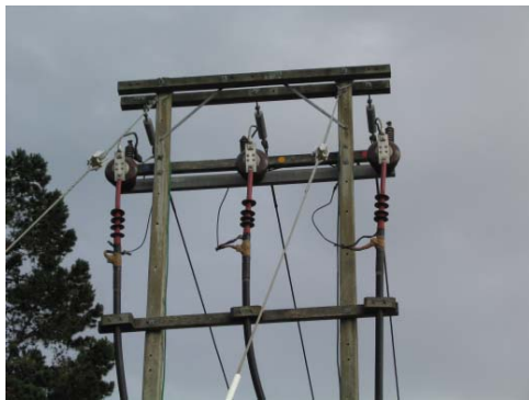
Fig. 1. The 3 -1/c XLPE submarine cables at Onerahi end
