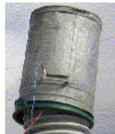
Figure 1- A set-up on a bushing head for interference suppression
